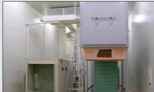
Air Volume Measurement Room
